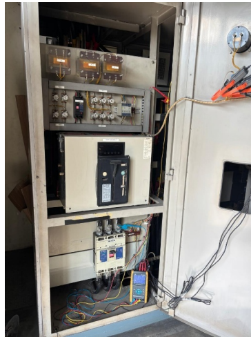
Figure 4. Injection Power Analyzer
