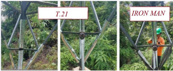
Figure 5. Iron Man on the Tower leg
