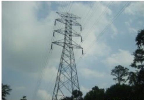
Figure 1. High Voltage Transmission Line (SUTT)
